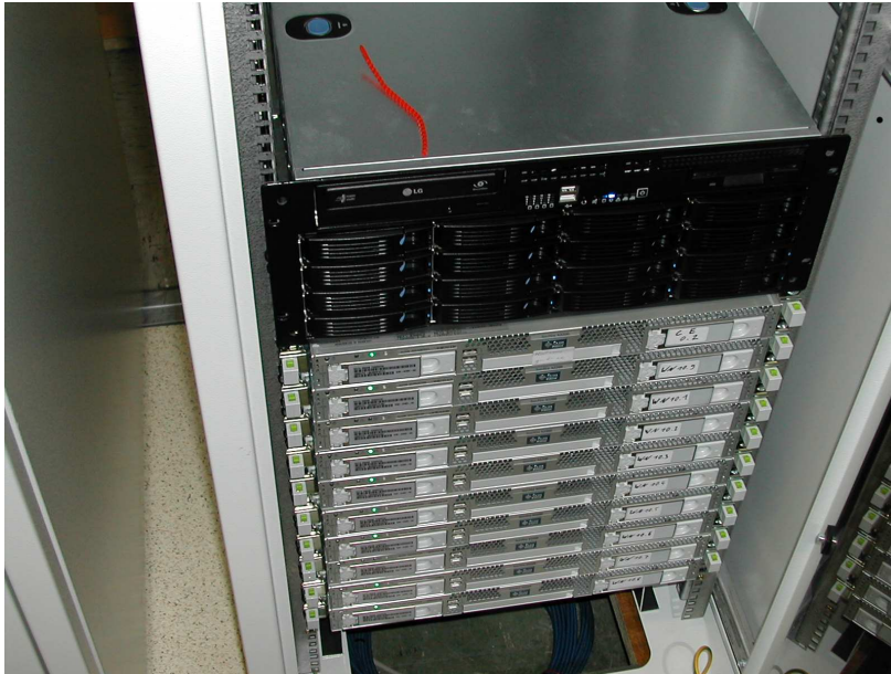
Figure 2: Photo of the SE , CE and WNs inside the 19" rack
